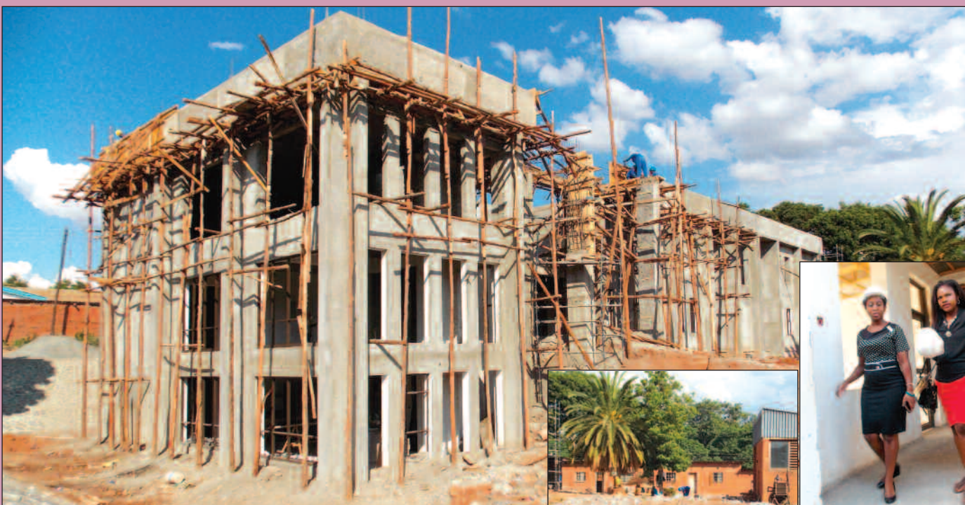
DoM offices under-going modernisation, inset are old offices. Far right is MGGSP's Temwani Gunda, in red, taking EU's Palamuleni through the Zomba, and Regional Geologist Office in Mzuzu.
