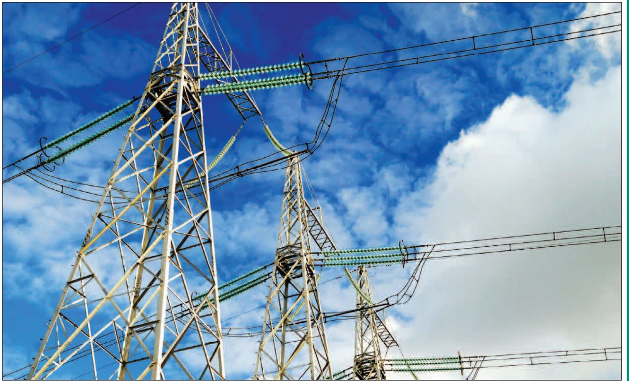
High voltage power lines
